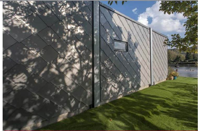
Dappled sunlight falls across the NedZink zinc shingles of the Amphibious House. Photo © Baca Architects
